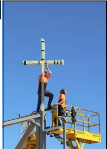
Above: Gungahlin Church construction work - midday. The completed church opened on 30 October as we went to print.
